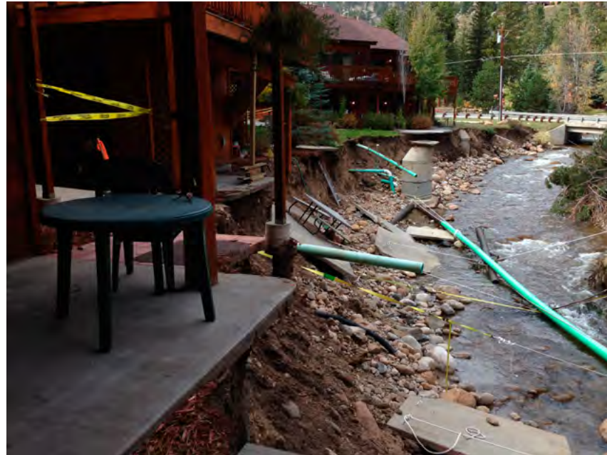
Estes Park Condos Antlers Point Utility and Structure Damage
